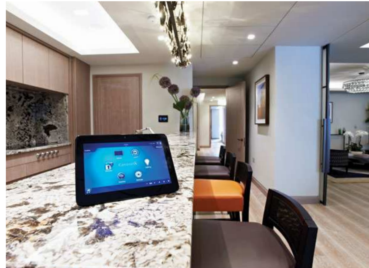
Every apartment features full Control4 integration and multiple touch screens.
