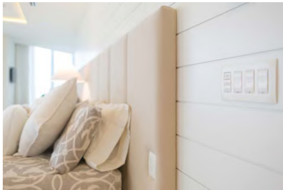
The master bedroom’s projection screen lowers on command and disappears into the ceiling when not in use. Clever keypads are built into bed frames and other convenient corners.
