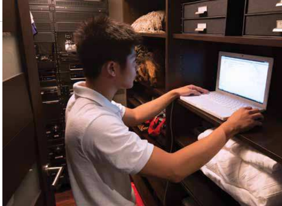
A custom installer programs motion sensors, Kwikset keypads and more in this Florida penthouse.
