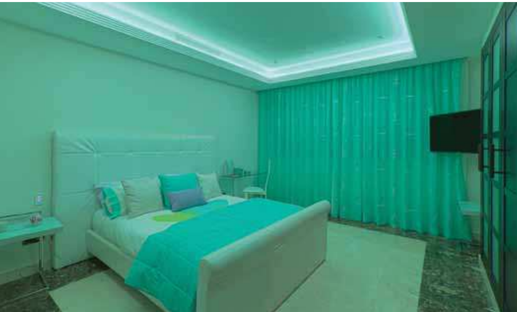
Unique LED lighting control dramatically changes the way rooms like the chillout room or bedroom can look or feel. All by the touch of a button or via a timed program.
